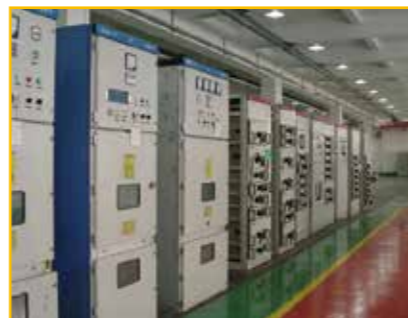
Electrical Engineering 电力电气
