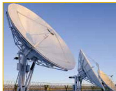
Telecommunication Station Base(TBS) 通讯基站
